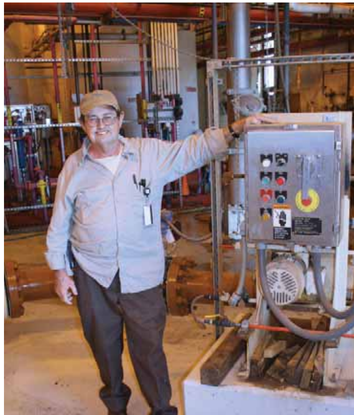
Cecil Chandler, the site's Operations and Management Technician with the Pipeline Lubrication System
